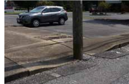
Utility pole in the middle of ADA ramp
