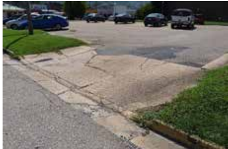
Deteriorated concrete entrance
