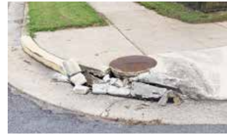
Busted concrete curb
