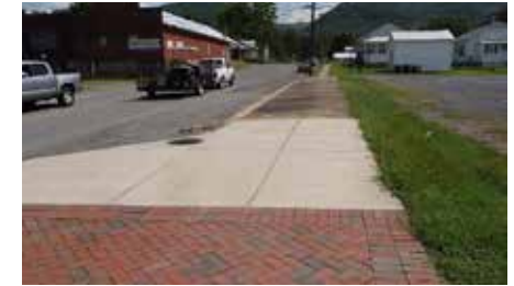
New paving materials end at old material
