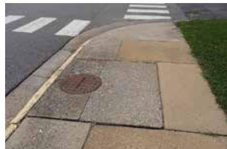
Concrete segments create non-level walkway surface that is a tripping hazard
