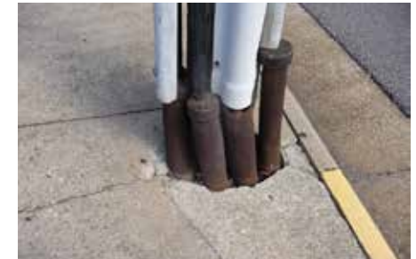
Unsightly utilities in walkway
