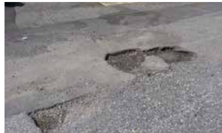
Large pothole in asphalt road
