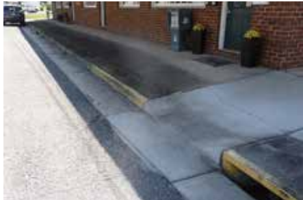
Curb ramp obstructs walkway, not ADA accessible
