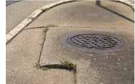
No curb ramps or crosswalk at street crossing
