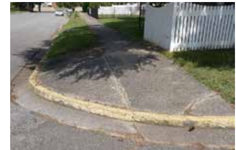
Steep sloping walkway down to curb not ADA accessible
