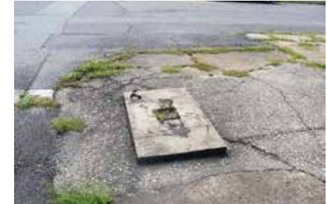
Old utility pedestal in walkway
