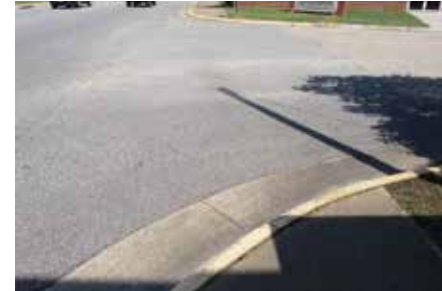
No curb ramps or crosswalks at intersections
