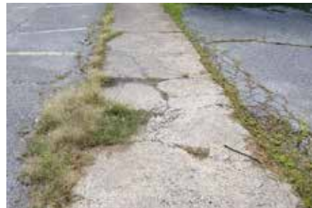
Cracks and grass in walkway
