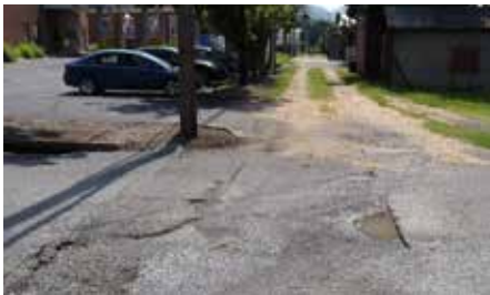
Holes, uneven areas and loose gravel in road, inconsistency in paving material with asphalt turning to gravel
