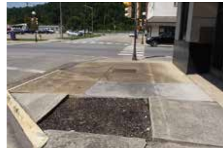
Vacant tree pit and heaving walkway
