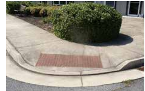
Curb ramp obstructs walkway, not ADA accessible
