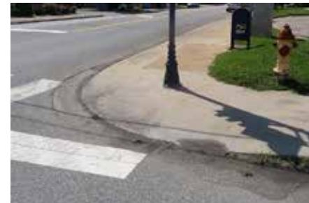
No ADA domes at curb ramp
