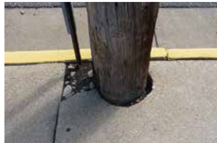
Gap around utility pole, busted concrete
