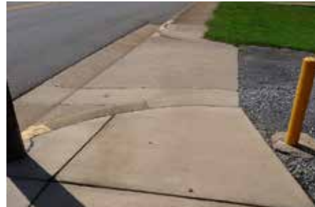
Drive entrance across walkway is not ADA accessible
