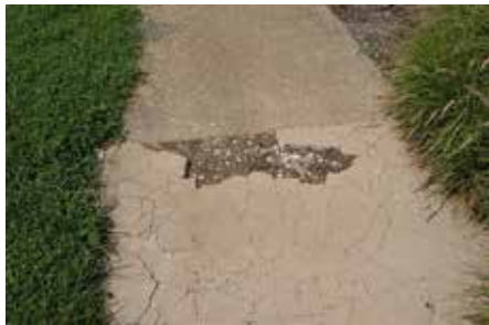
Hole in concrete walkway
