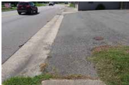
Asphalt from adjacent parking displaces concrete walkway
