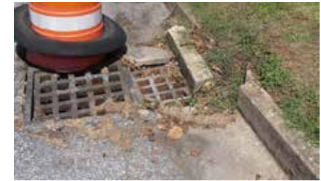
Busted concrete curb
