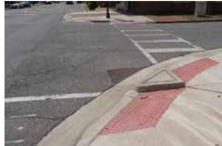
Faded crosswalk striping
