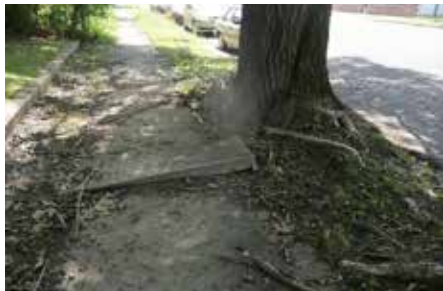
Walkway heaving and damaged from tree roots
