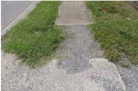
Concrete section missing in walkway
