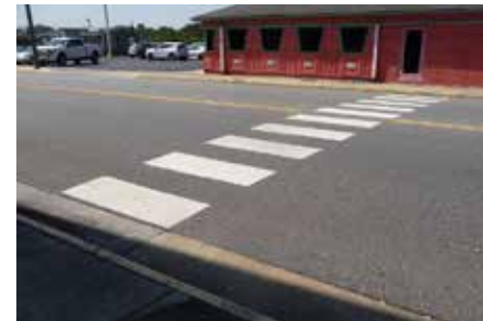
No curb ramps at mid-block crossing
