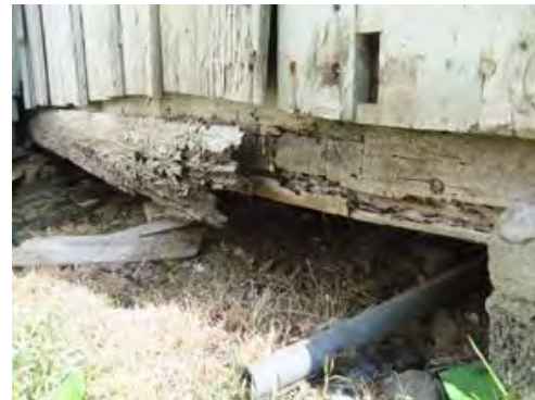
Figure 30: Sill Beam Deterioration
