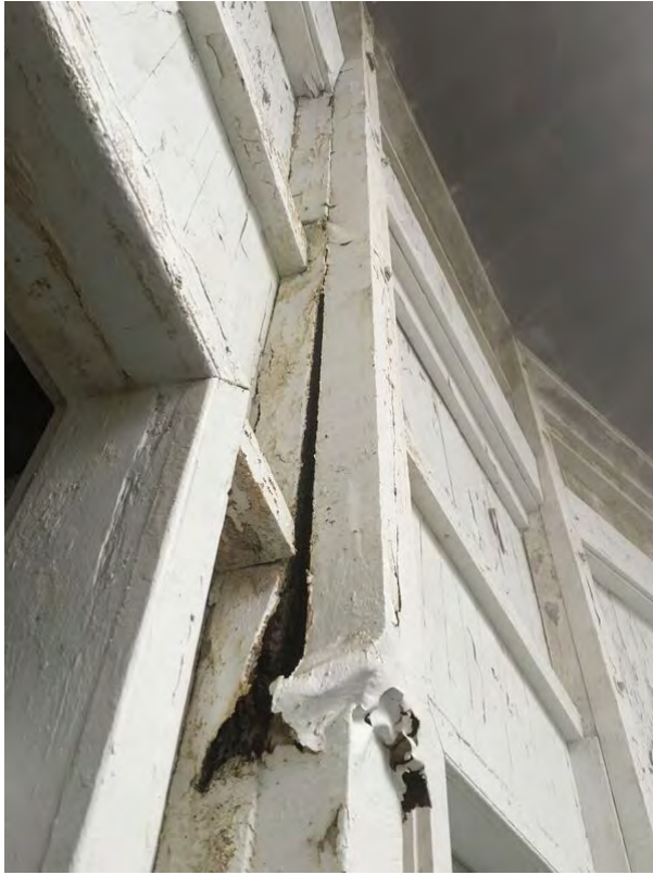
Fig 126. Inner ring structure buckling and showing moisture damage.
