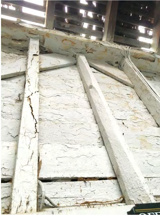
Fig 100. Moisture damage at south wall
