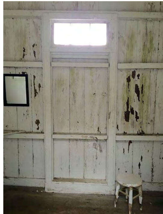
Fig 127. Interior of typical dressing room on south side showing former door opening.
