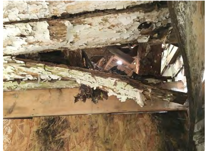
Fig 113. Deterioration at the junction between the East Wing and the Southeast Addition.
