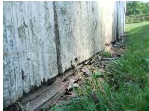
Figure 27: Perimeter Sill Deterioration
