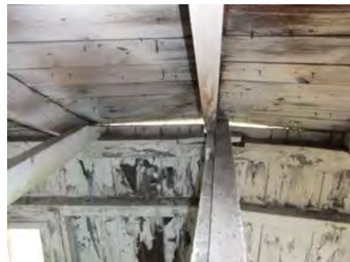
Figure 17: Separation of splice at outermost wall top plate.
