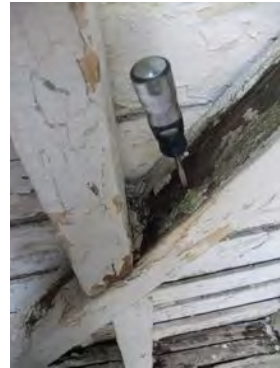
Figure 39: Wall Brace Deterioration
