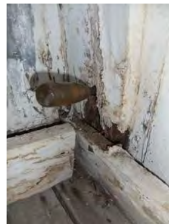
Figure 15: Rotting post base
