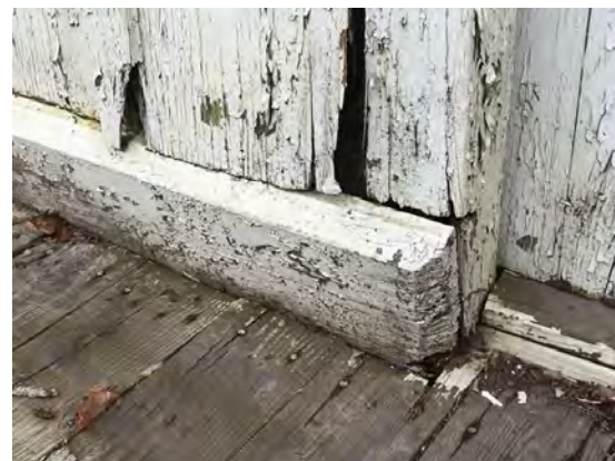
Fig. 122. Condition of the lower wall on the northwest.
