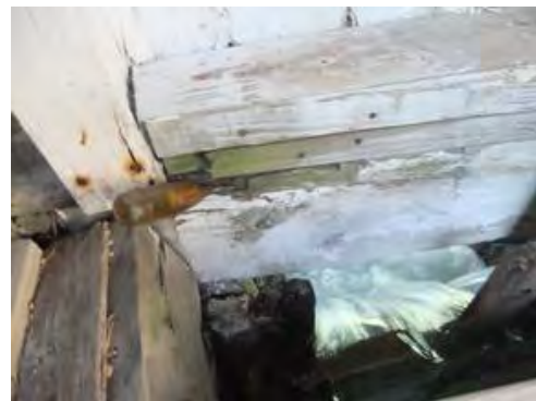
Figure 14: Rotting sill beam over spillway
