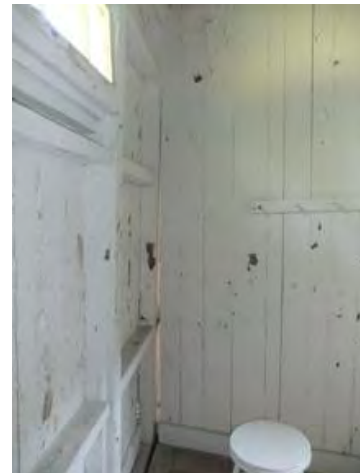
Figure 18: In-plane wrinkling of tongue and groove partition walls
