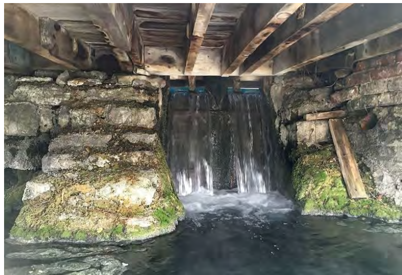
Fig 117. Outflow from the Ladies' Bath showing stone buttress to left and brick spout bath enclosure to the right.
