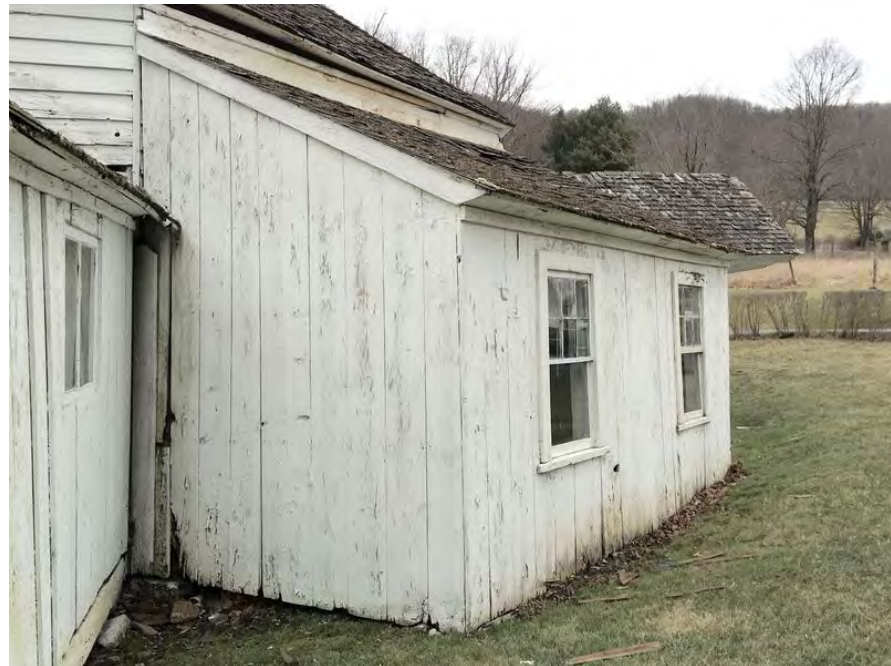
Fig. 115. Northeast wing from the east. Note how the slipped roof at the top has dropped.
