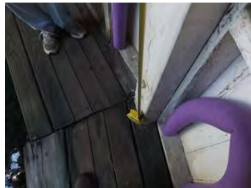
Figure 16a & 16b: Lateral displacement of posts
