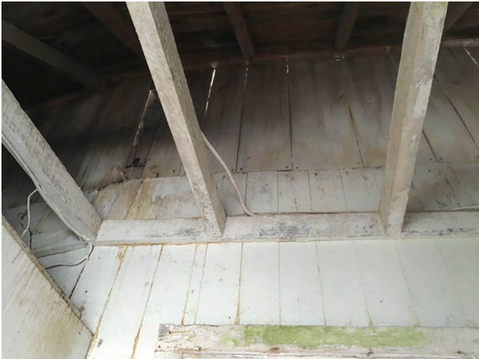
Fig 128. View from dressing room showing original upper sheathing and replaced lower sheathing on inner ring
