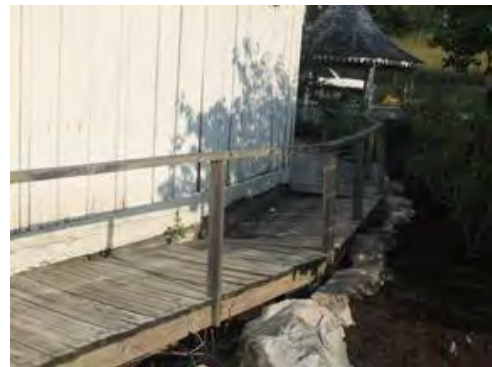
Figure 6: Deck Walk Deterioration
