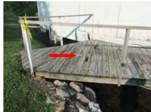
Figure 7: Deck Walk Deterioration
