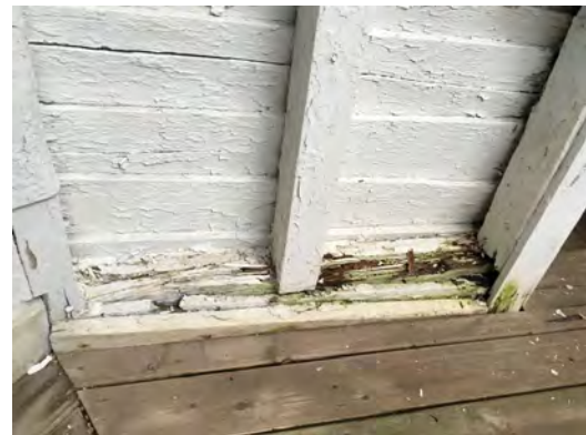
Fig 101. Moisture Damage at replaced sill on east wall
