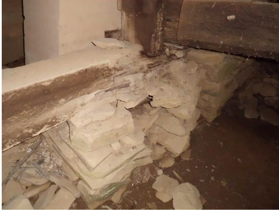
Figure 44: Hurst frame bearing deterioration and looseness in masonry below
