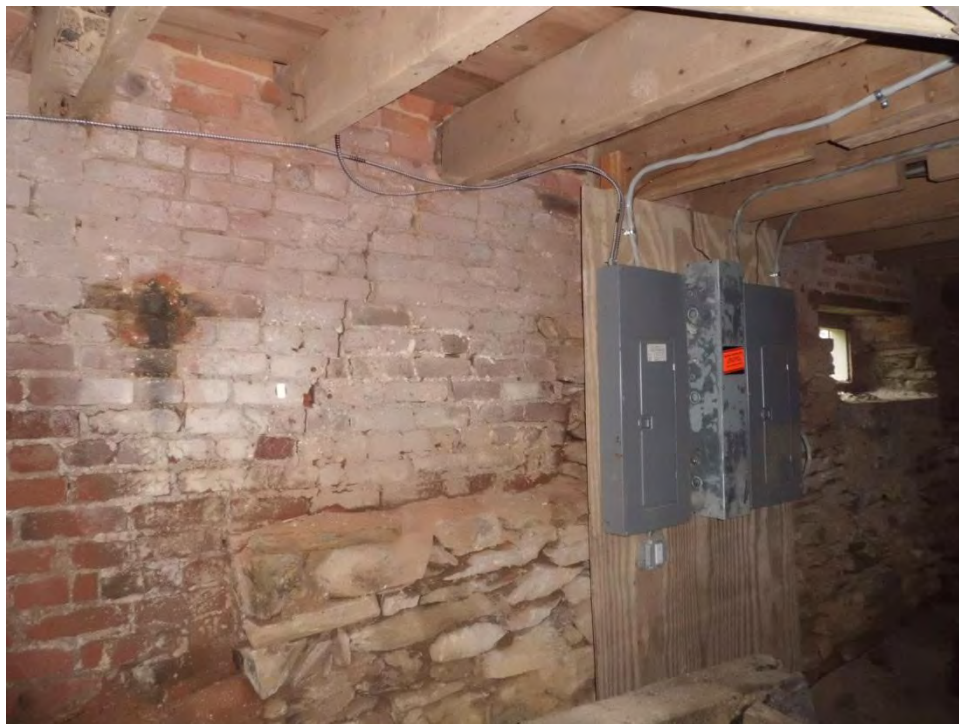
Figure 47: Vertical crack in brick masonry above stone foundation wall at northwest corner
