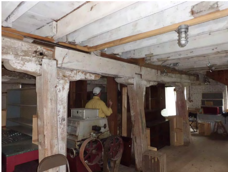
Figure 24: Second floor longitudinal beam sister reinforcement. Note misalignment of post above and post below at left.
