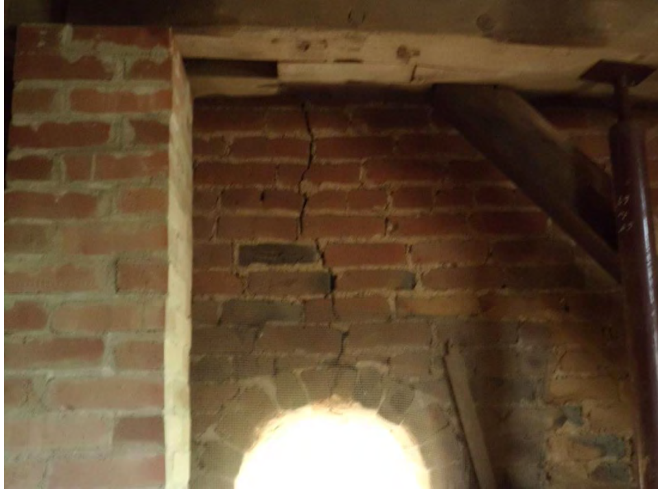
Figure 46: Vertical crack in masonry at west window of south elevation
