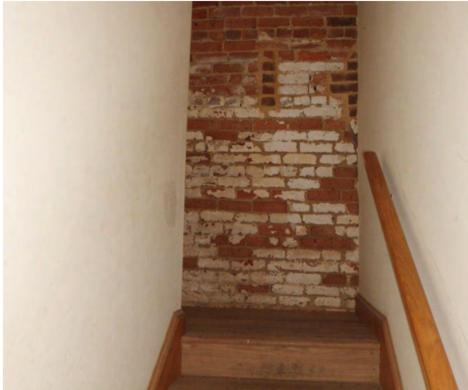
Figure 31: Brick spalling within northwest stairwell landing
