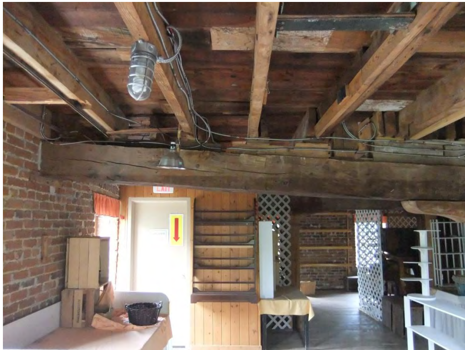
Figure 18: Third floor beam deflection
