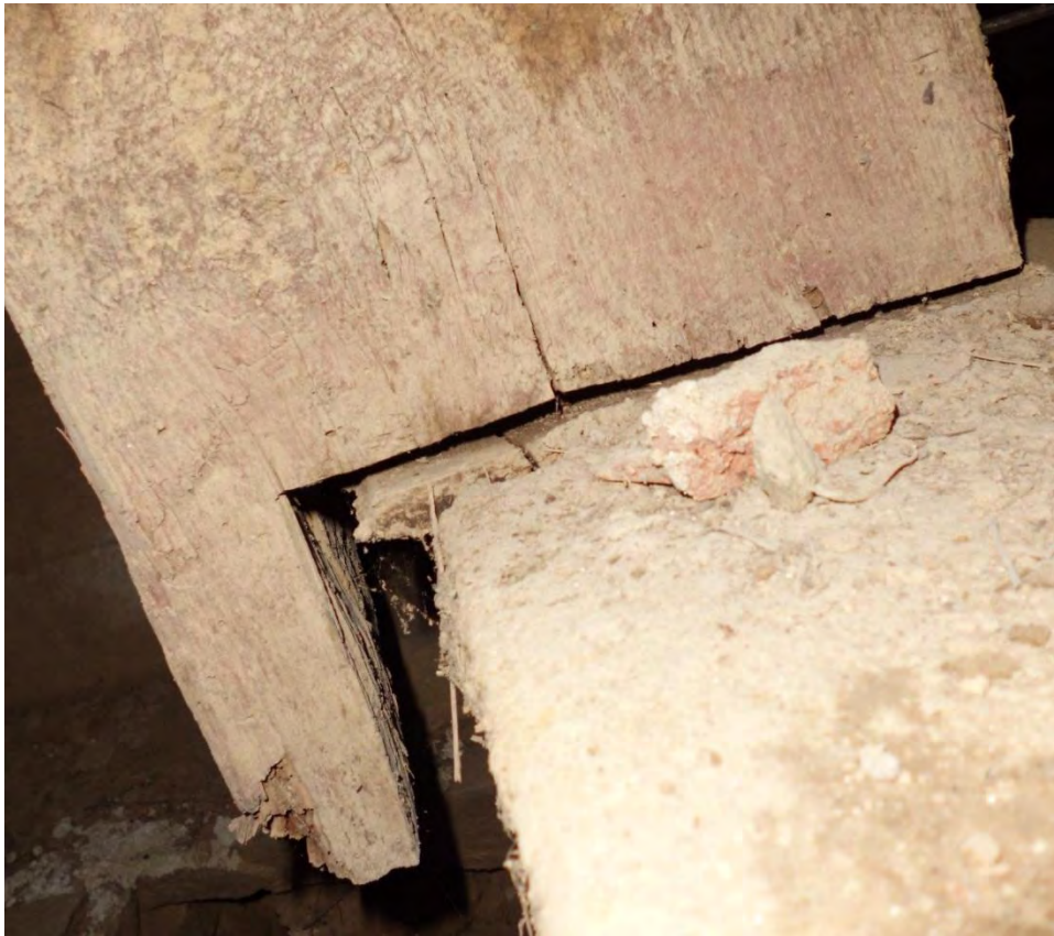
Figure 42: Canted brace bearing deterioration on Hurst frame
