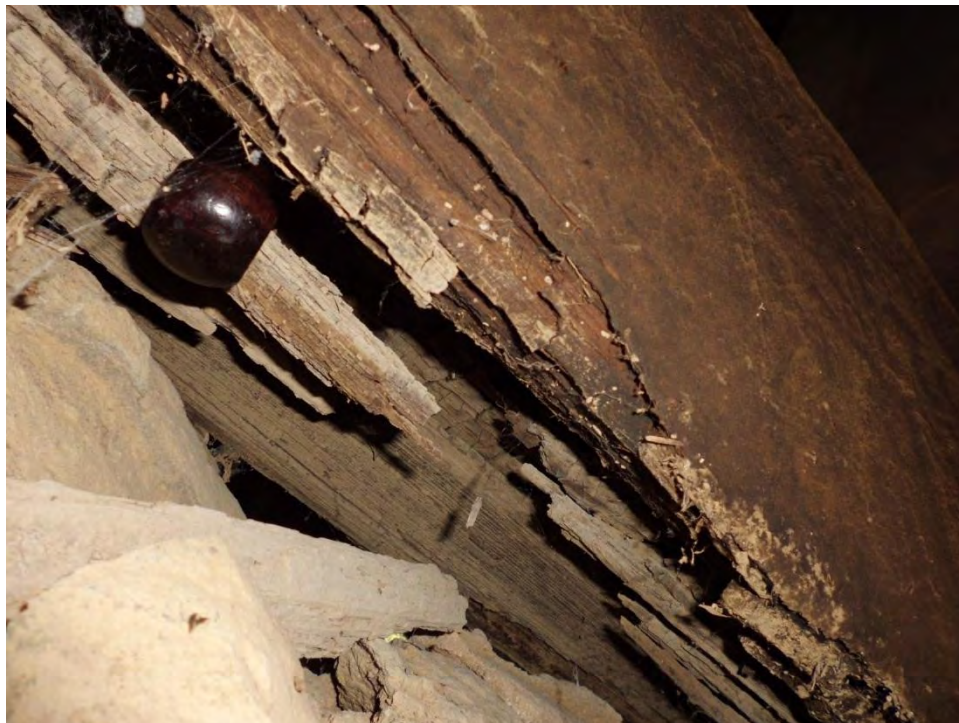
Figure 45: Hurst frame deterioration
