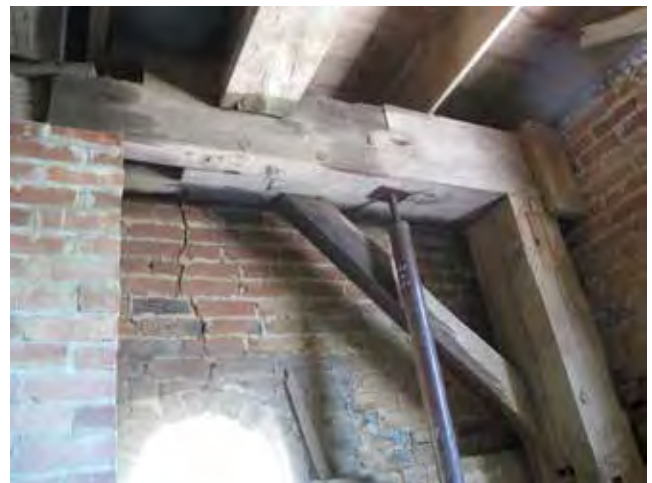
Southwest corner post seen from northeast showing surviving brace
