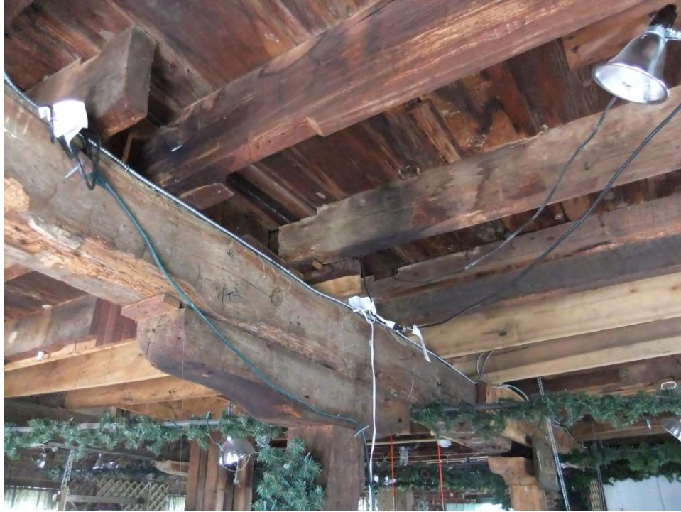
Figure 9: Attic joists on longitudinal beam below. Note leveling shim pack and column capital.
