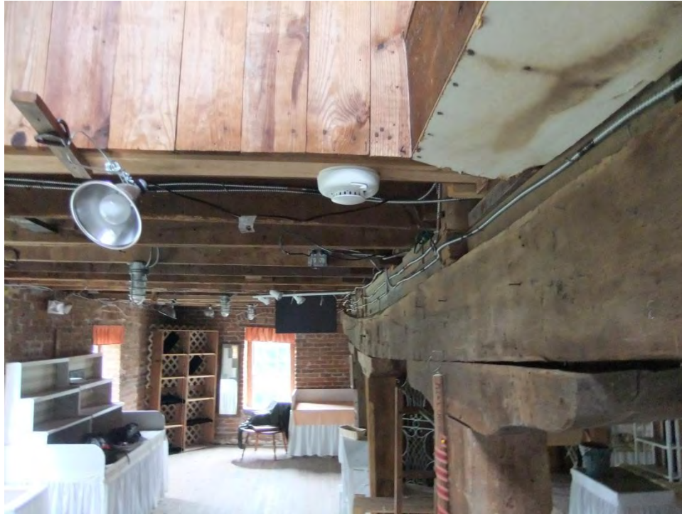
Figure 17: Third floor beam deflection
