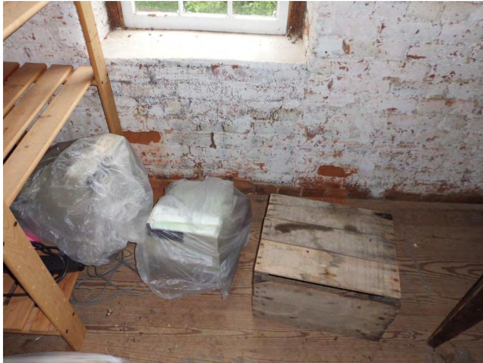
Figure 29: Spalling of masonry below first floor window opening along south wall
