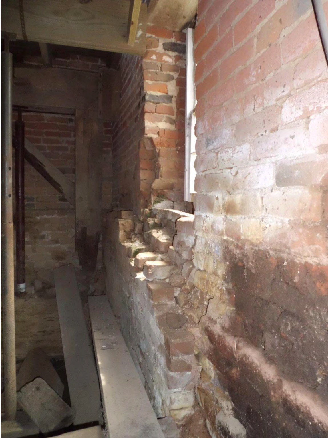
Figure 49: Deterioration of brick masonry at southern window of west foundation wall
