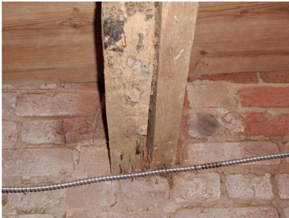
Figure 36: First floor joist bearing deterioration at northern masonry wall
