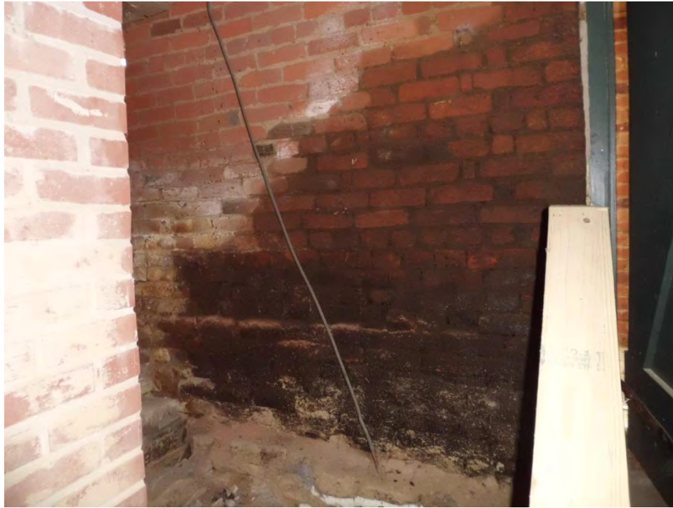
Figure 48: Saturation of brick masonry above west foundation wall
