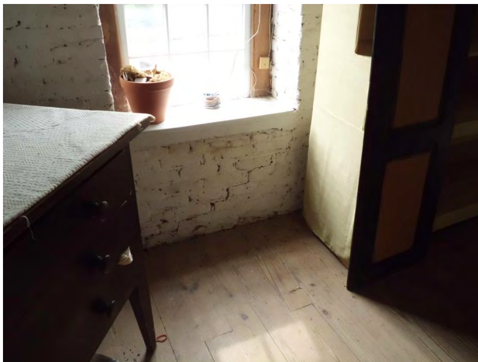
Figure 30: Diagonal cracking within mortar joints below first floor window opening along west wall
