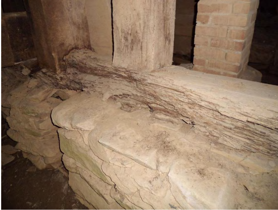
Figure 41: Canted brace with deteriorated Hurst frame support
