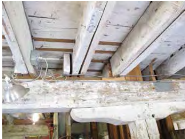
The southeast post on the first floor, showing typical blocking and sistering performed in 1983-4.
