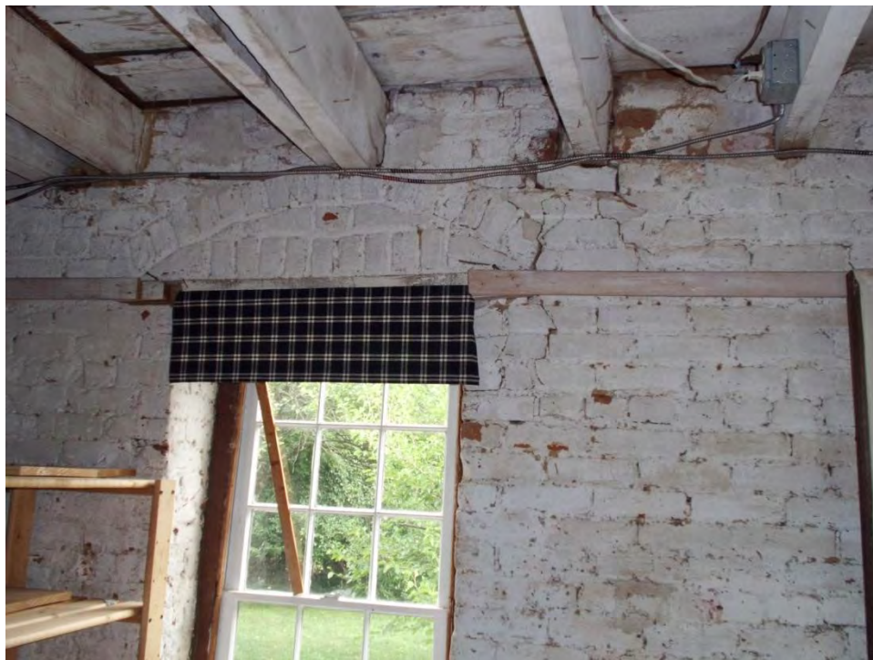
Figure 32: Second floor joist bearing deterioration at exterior masonry pocket
