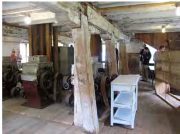
First floor looking east from south structural bay showing added braces and roller stands.
