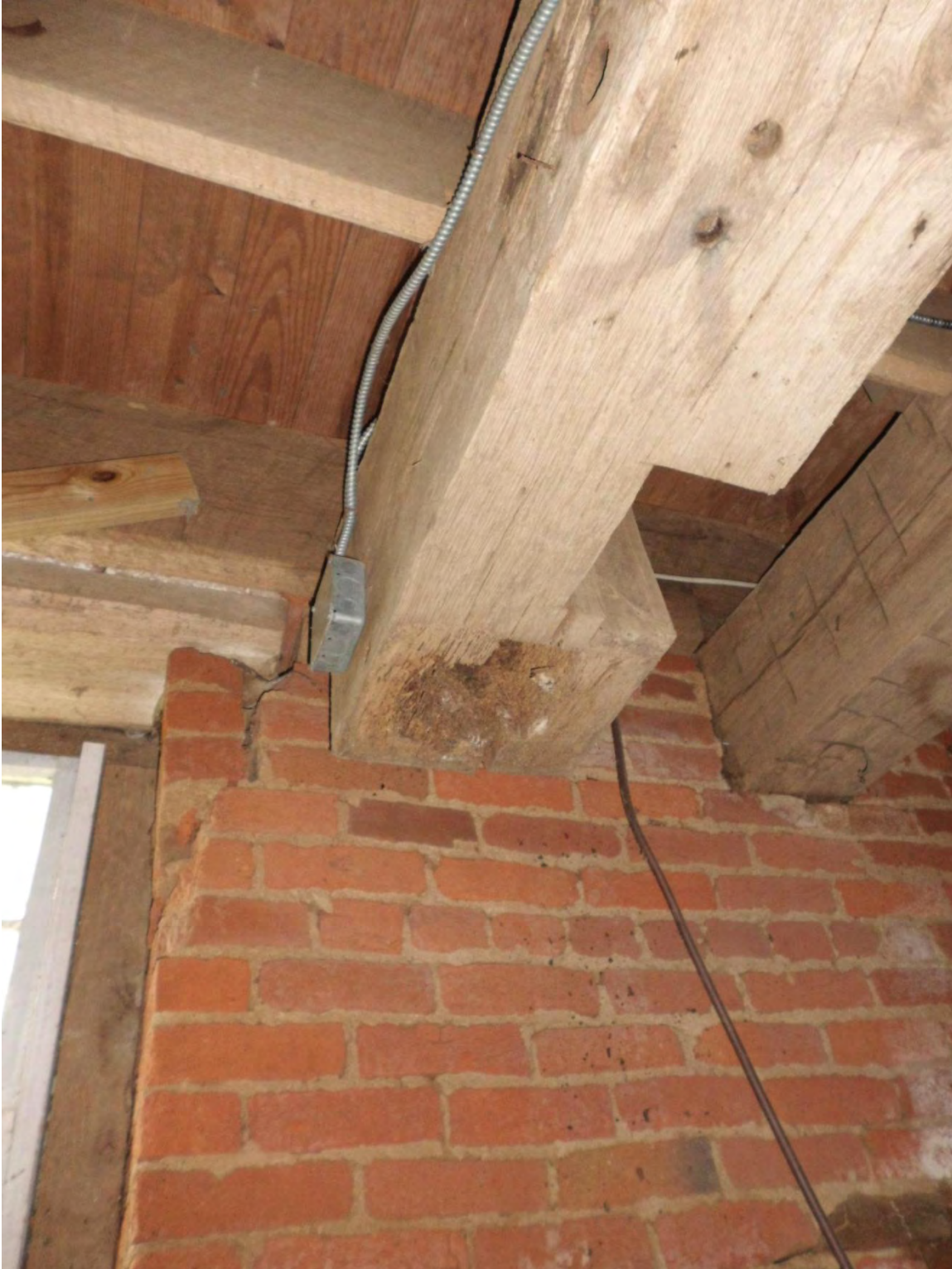
Figure 43: Hurst frame beam with loss of supporting post and cracked masonry at opening to left
