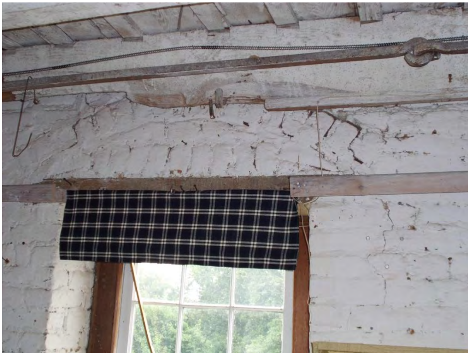
Figure 28: Cracking in masonry above first floor window along west wall
