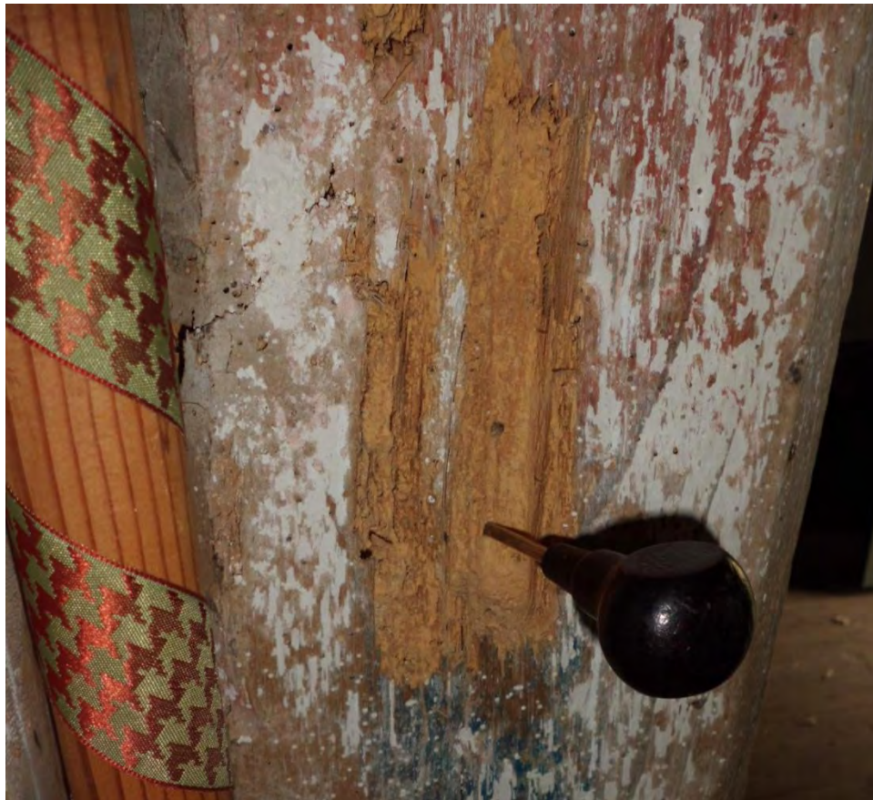
Figure 26: Second floor southeast corner column deterioration
